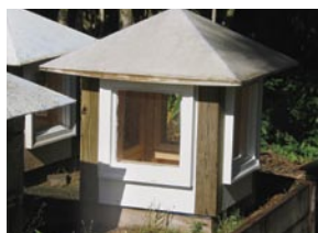
AuraLast wood was put to the test for several years in a very harsh and humid environment.
